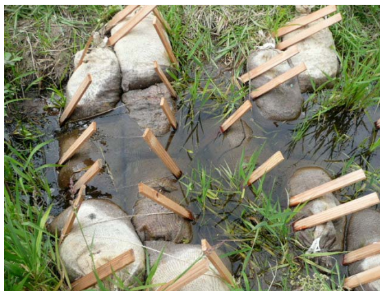
Ecler mycoremediation installation
