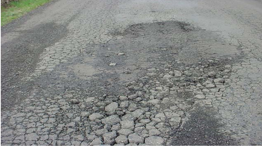
The above photo shows road damage caused by heavy vehicles during a freeze/thaw event.
